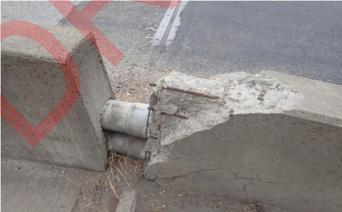
Damage to bridge rail at southwest corner looking east.
