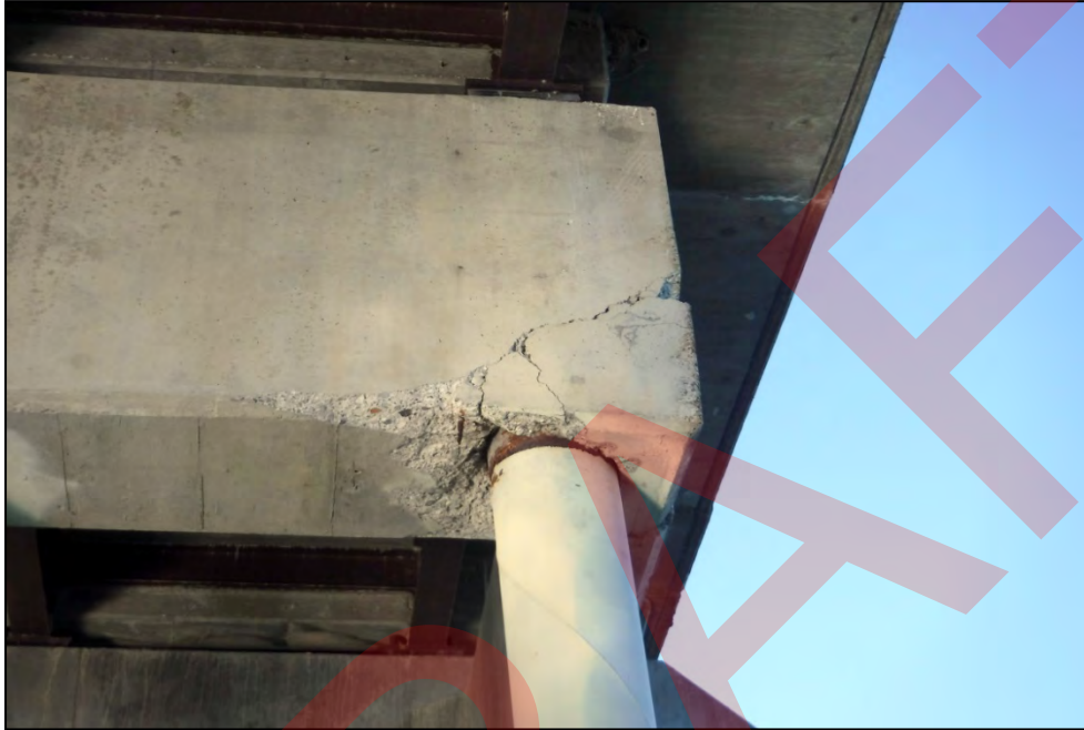
Photograph 7: View of Cracking and Section Loss at Southeast Corner of Tower 3.
