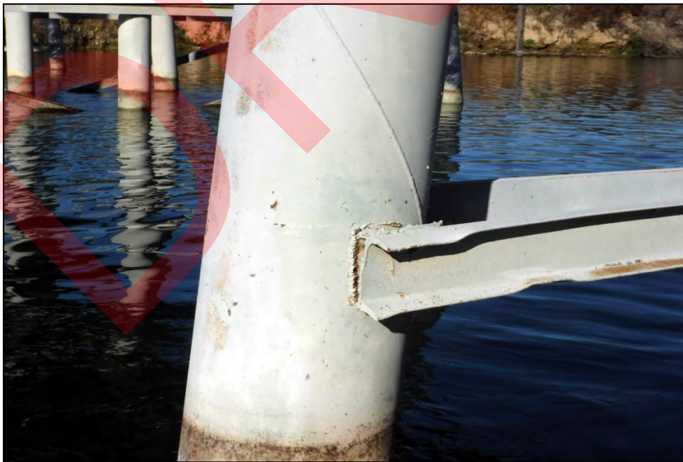
Photograph 6: View of Broken Horizontal Brace Connection at Bent 16, Looking Northeast.
