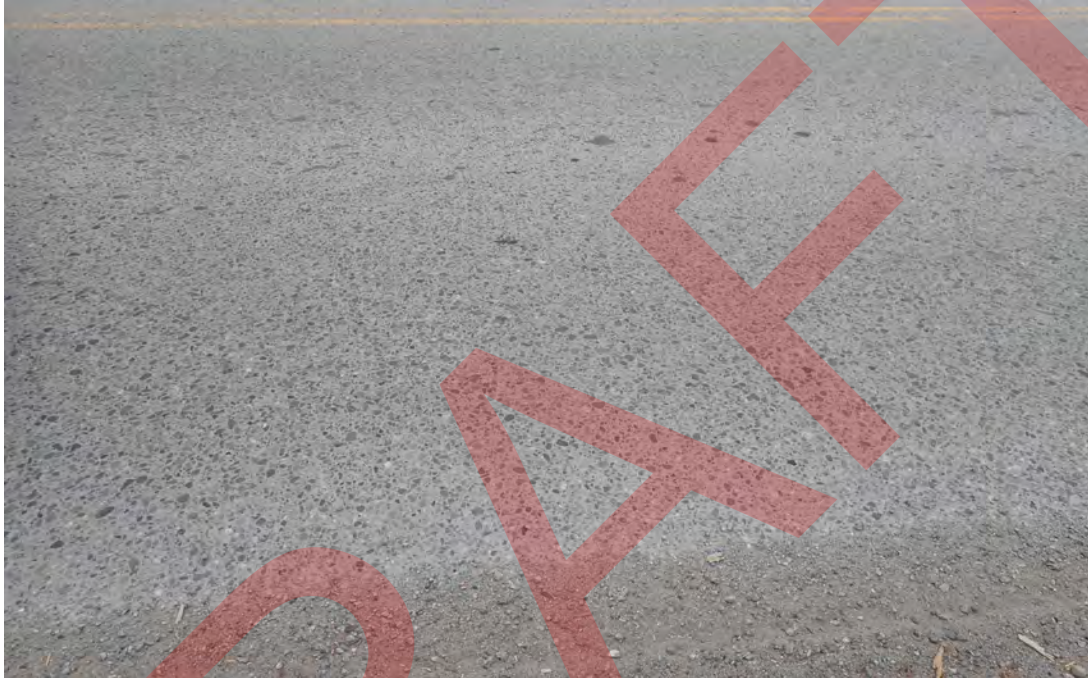
Typical abrasion in the top of the deck.
