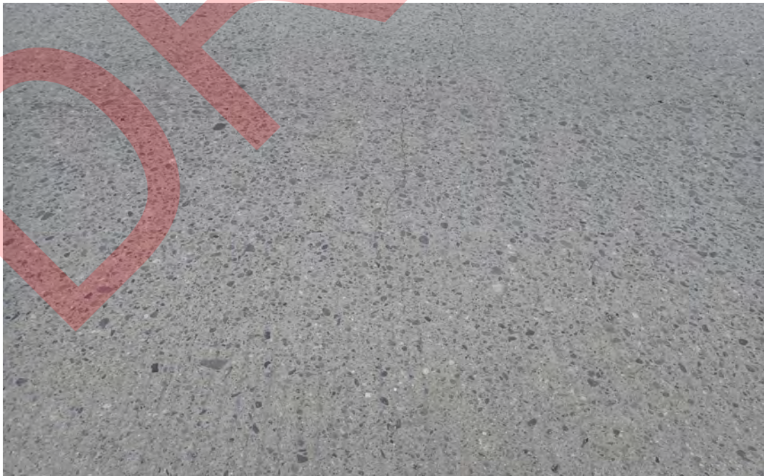
Typical cracking in the top of the deck.
