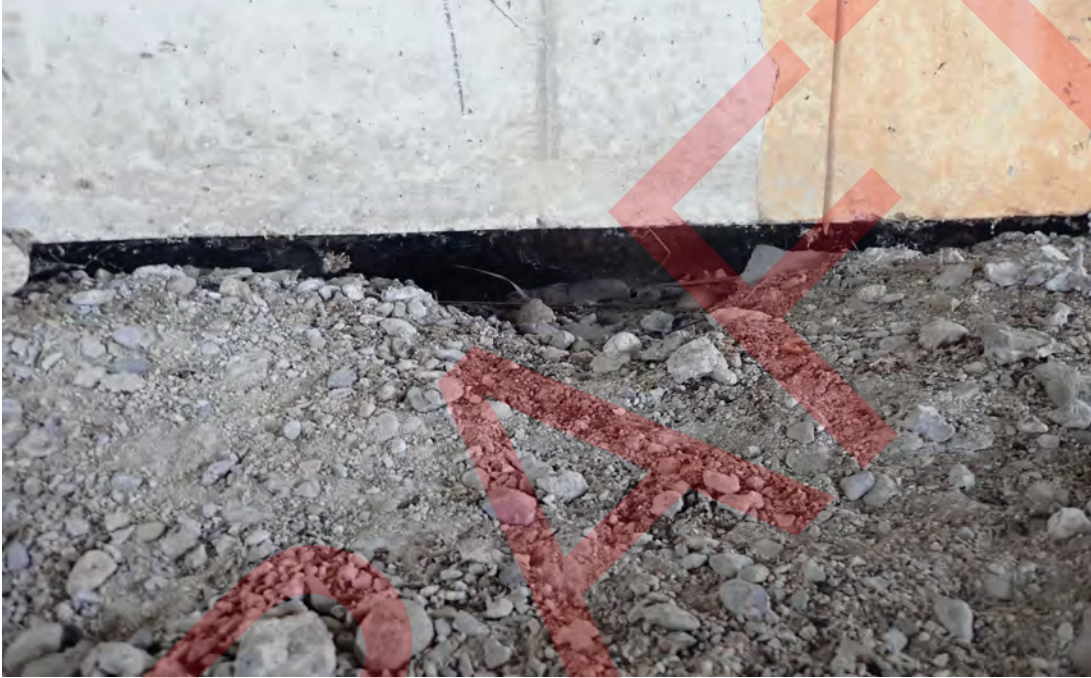
Erosion and undermining at the south abutment.
