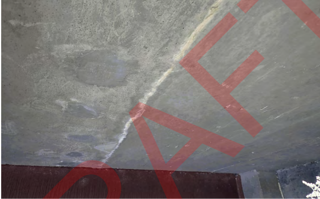
Typical cracks with efflorescence in the deck underside.
