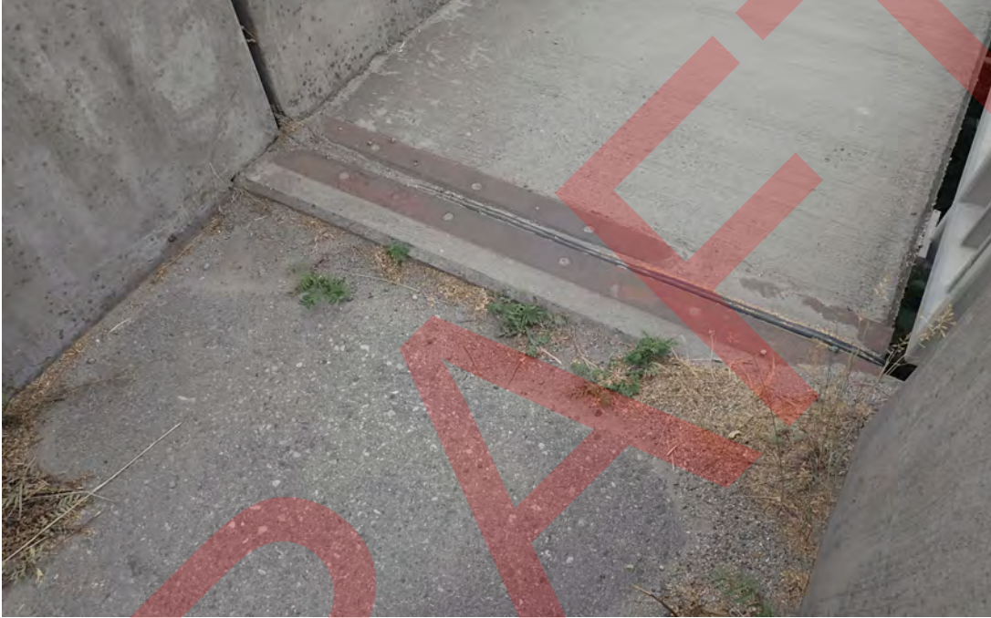
Settlement in sidewalk at north approach.
